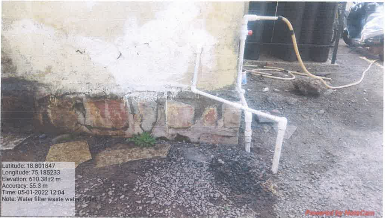
Water filter waste water outlet
