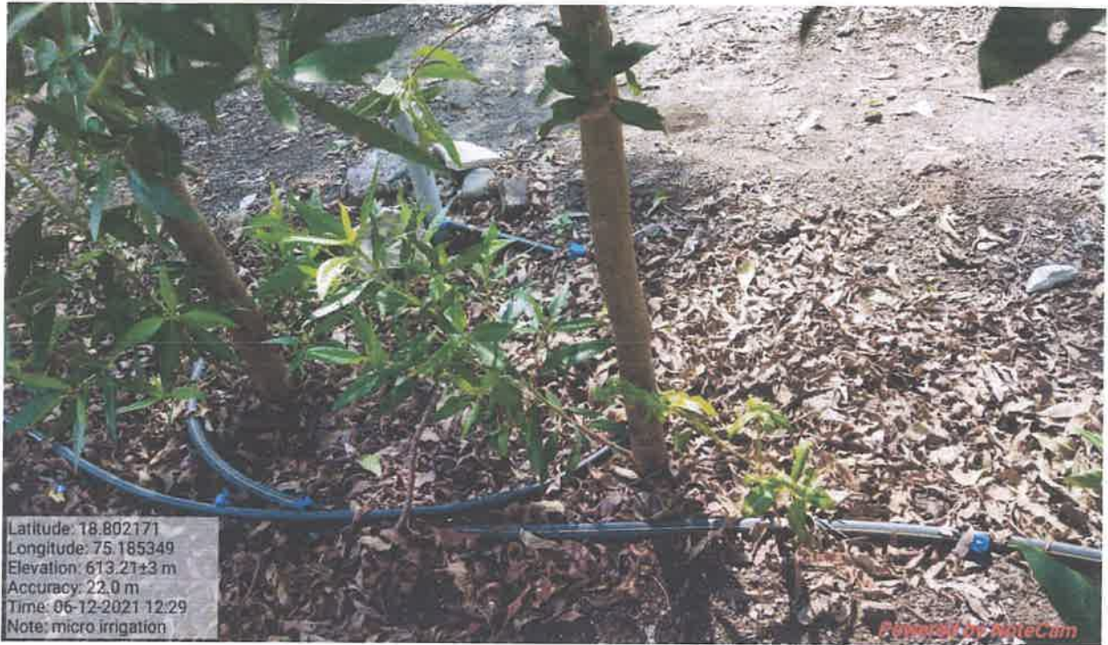
Micro irrigation System
