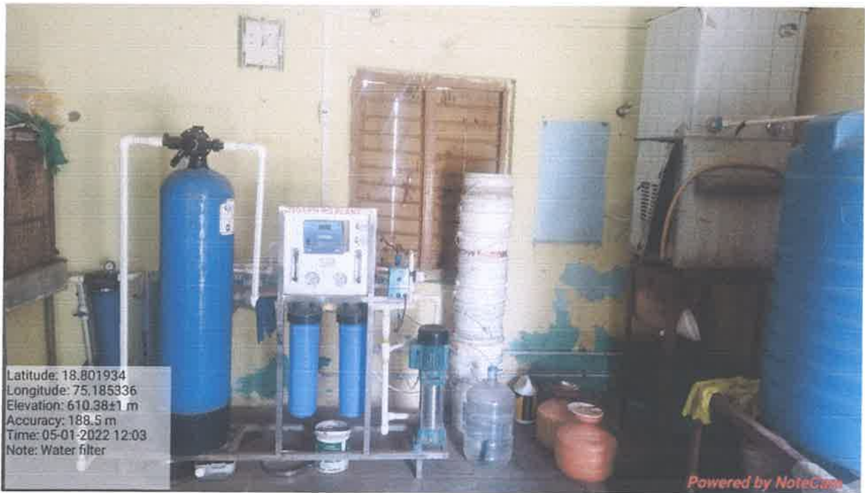
Recycling of Waste Water from Water Filter to the plants in the campus
