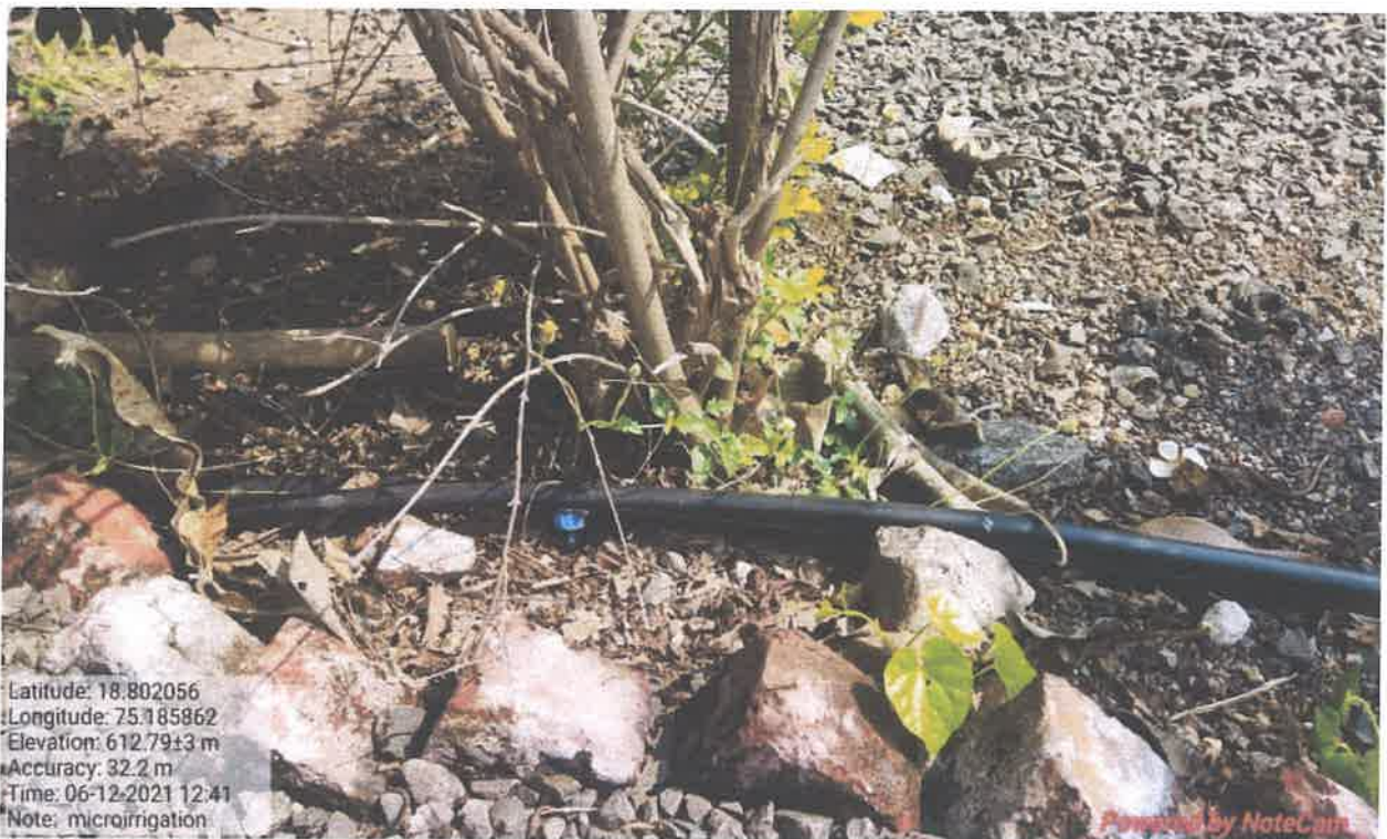
Micro irrigation System
